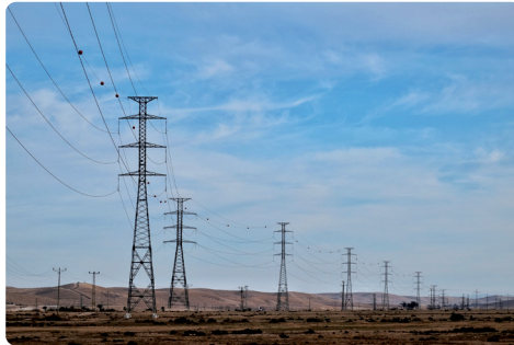
Electricity generated in power plants are distributed to homes through power lines.
