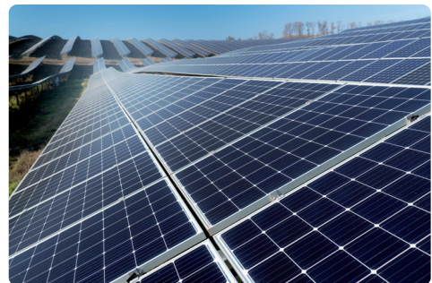
A solar energy farm
